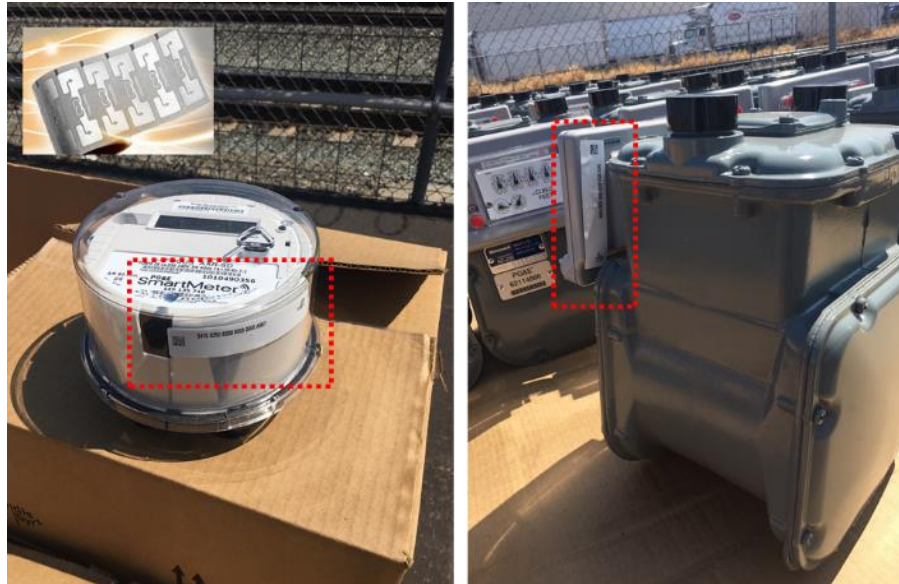
Figure 20: RFID Tags on Electric and Gas Meters
