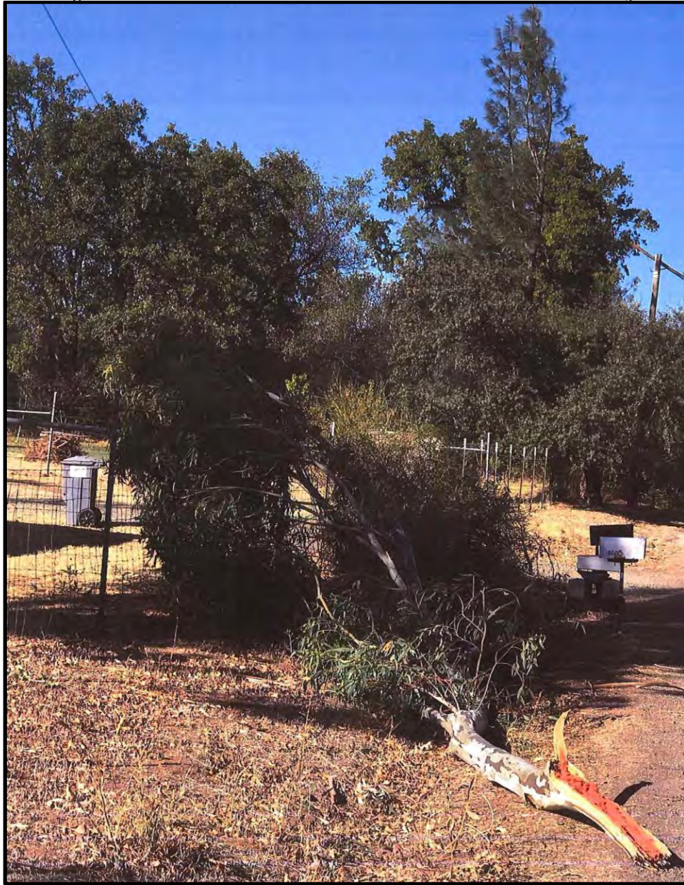
Figure 4: Tree fell, broken conductors; Oroville, Butte County
